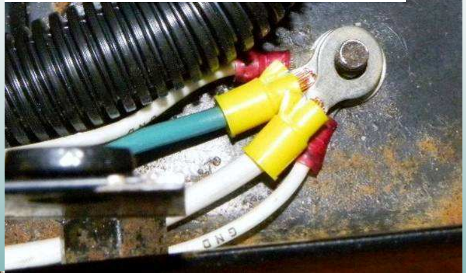
Neutral & 120v Grounds + Onan circuit grounds
